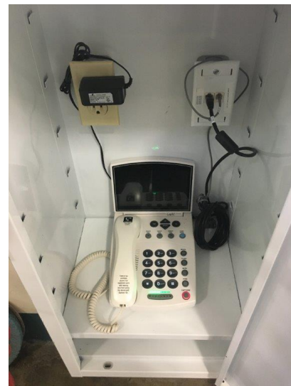
Captel, inside cabinet
