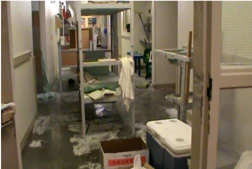
Caption: Photo of destruction of MSU unit during disturbance
