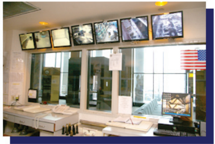
The Nashua Street Jail control panel
