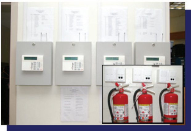
The En-Gauge monitoring system
